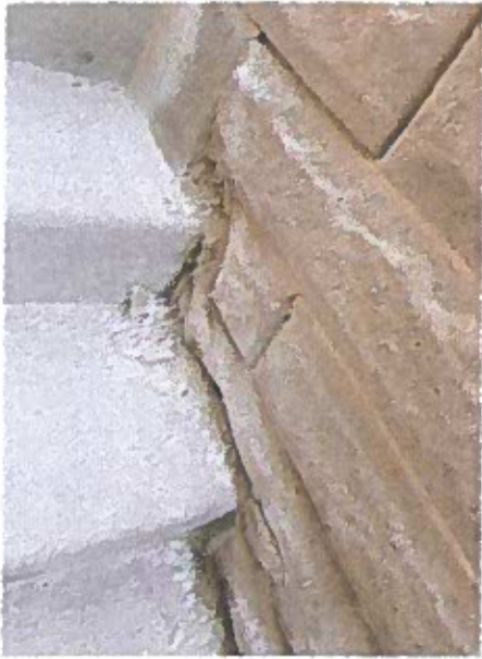
Unnatural deterioration of stairs. Appear to be "dug/picked at"
