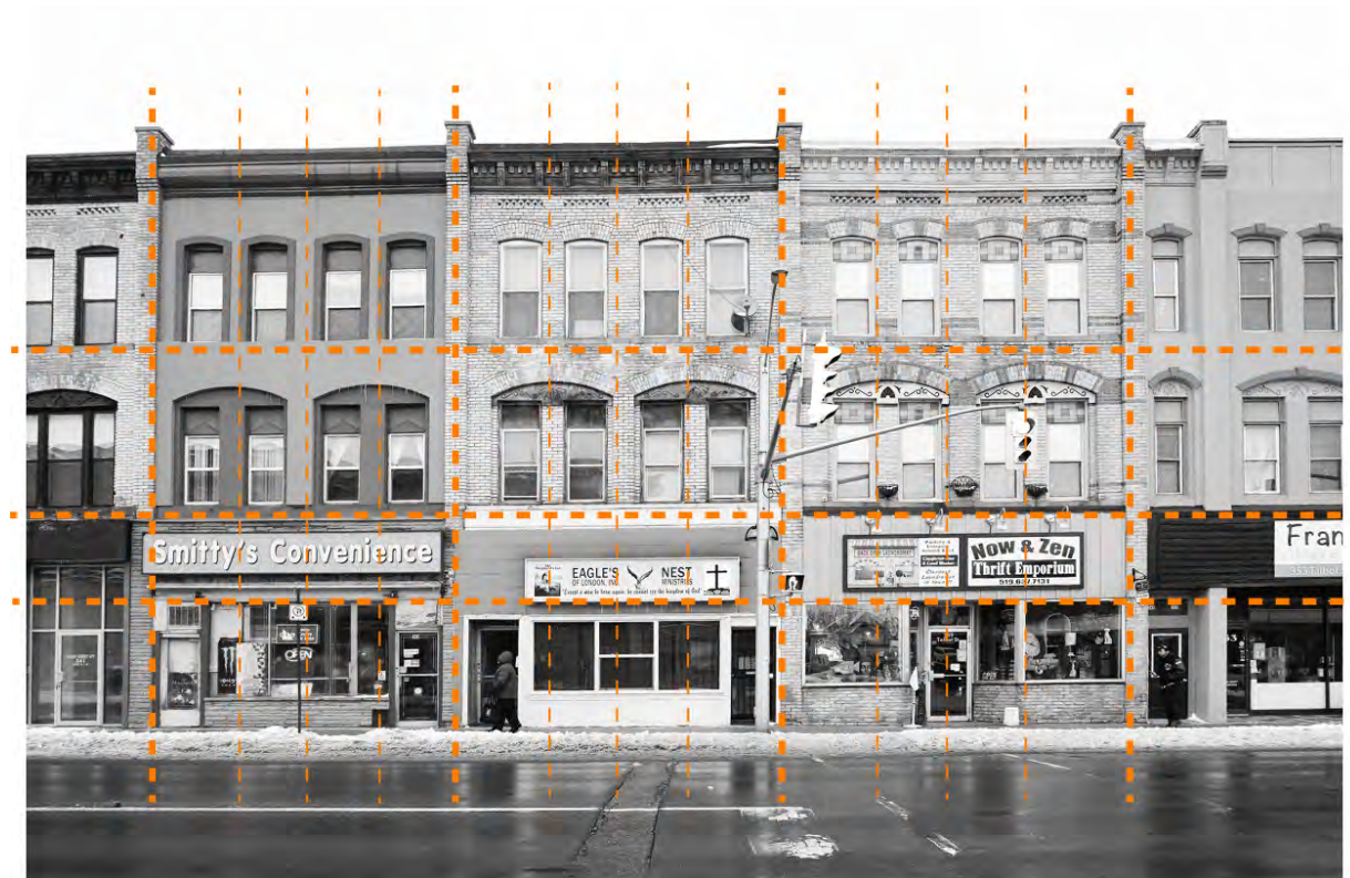
Plate 5: Maintain the rhythm of windows and doors in the façade that make up the traditional commercial/mixed-use façade pattern in the HCD
