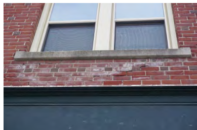
Efflorescence under window due to improper water drainage can cause damage to masonry. Consider methods to reduce water damage.
