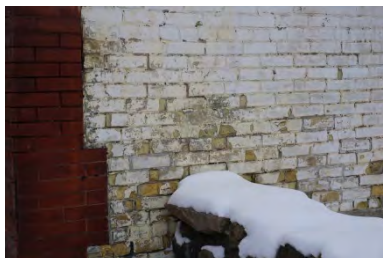
Paint in bad condition on a side of a building, the brick underneath is in very bad condition.
