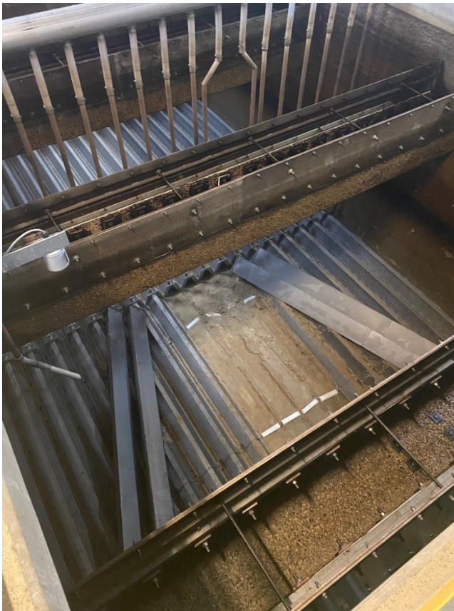
Figure 5: Filter #2 pre-repair. The filter media (anthracite and sand) was removed to inspect the filter. Four (4) underdrains are set aside revealing filter
