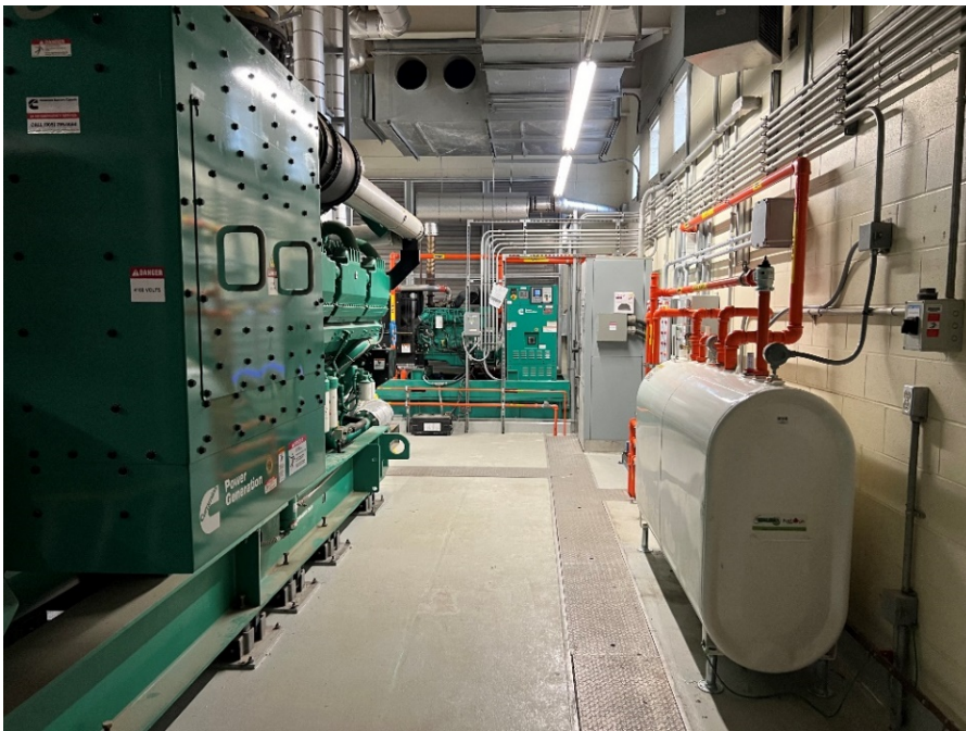
Figure 7: View of the 2.5 MW generator and associated fuel day tank, with the smaller 100 kW generator in the background.
