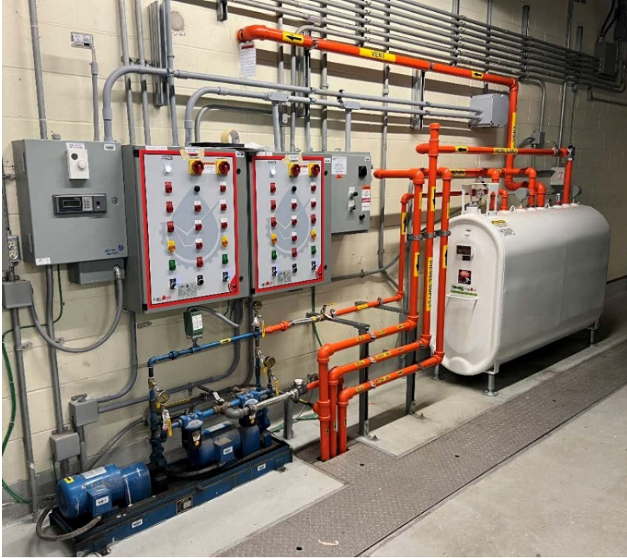
Figure 6: New fuel day tank, diesel transfer pump control panels, and associated piping.
