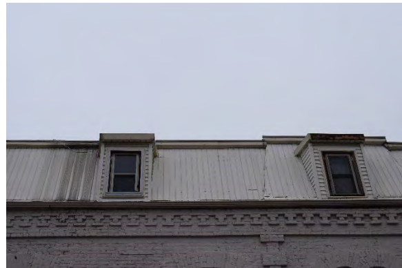
Plate 23: Details of mansard roof, dormers, and corbel on 248 Talbot Street, looking west
