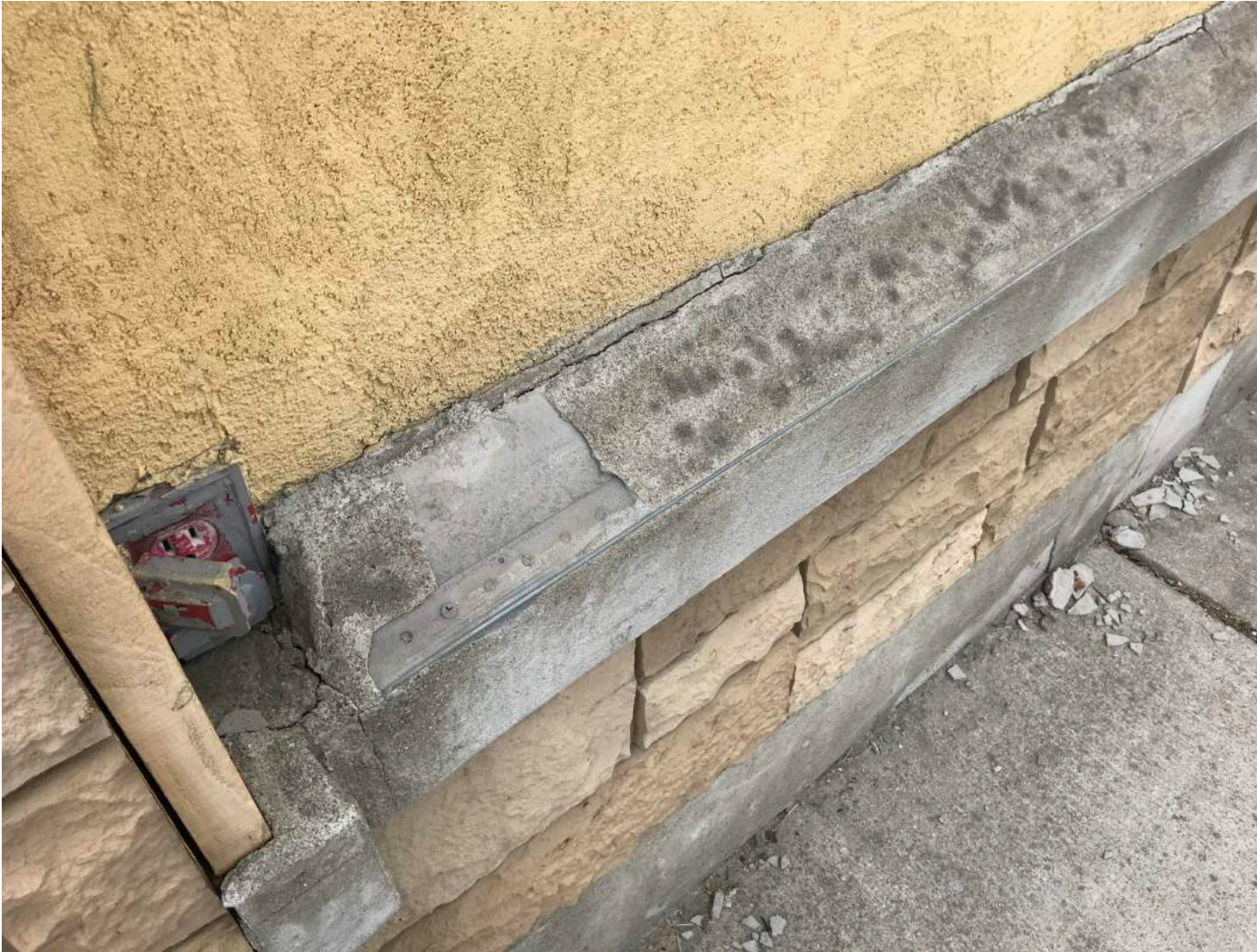
Example of missing parging along facade of Destination Church - Photo Taken June 29, 2021
