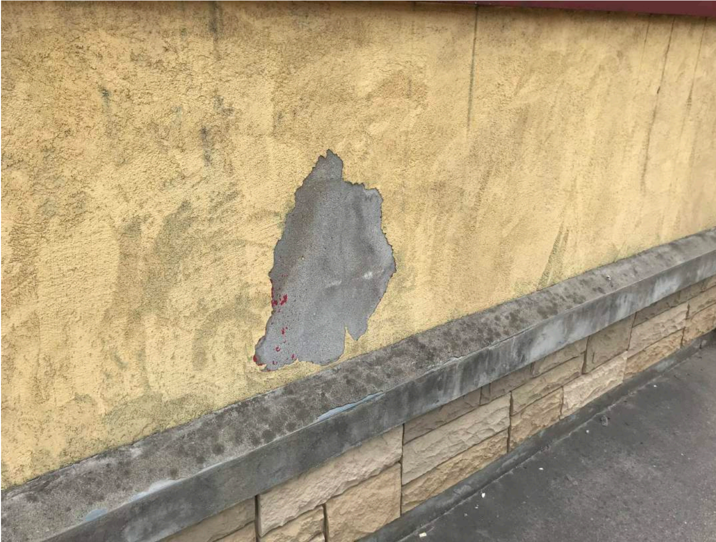
Further example of facade deterioration at Destination Church - Photo Taken June 29, 2021
