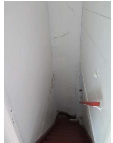
4.3 PEELING AND BUBBLING PAINT IN CHOIR BALCONY STAIR AREA
