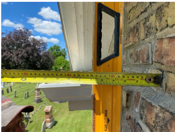
Out of Plumb Measurement Displacement ranges from 2" – 3"
