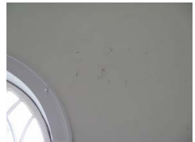
4.6 CRACKED PAINT BETWEEN WINDOWS
