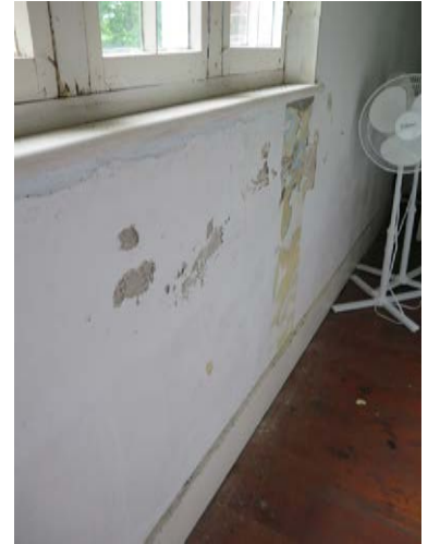
4.4 PEELING PAINT AND WALLPAPER ON EAST WALL IN TRANSEPT
