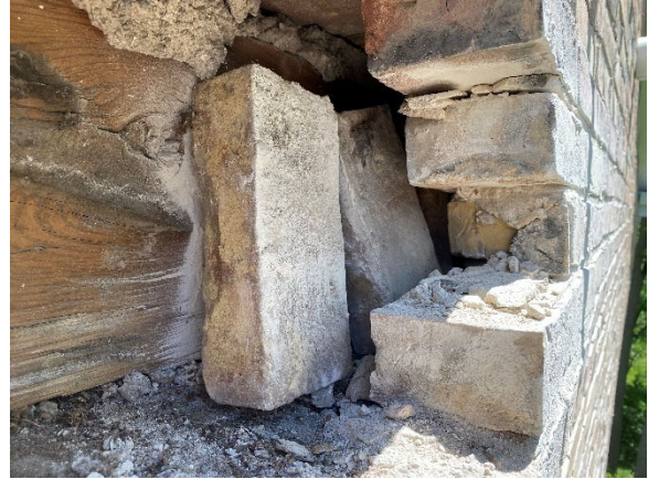
Opening Detail Loose masonry removed
