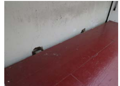
3.2 GAP BETWEEN CHOIR BALCONY AND SOUTH WALL
