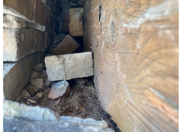
Void Space Loose laid brick infill and mortar debris.
