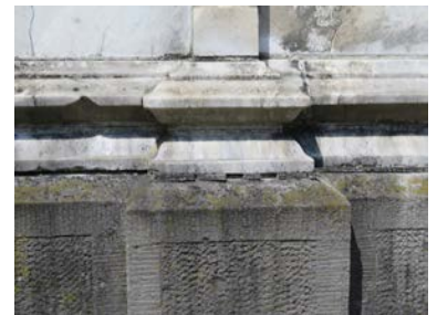
9.4 OPEN JOINTS ON CHISHOLM MONUMENT
