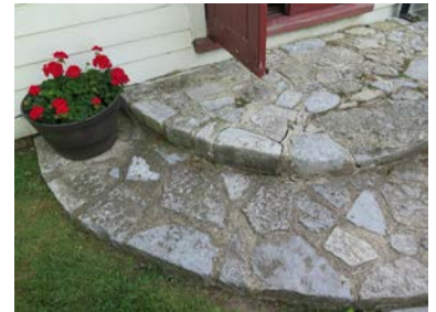
2.2 LOOSE STONES AT THE MAIN ENTRANCE STEPS
