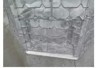
8.1 RUST ON SPIRE SHINGLES AND MISSING PANEL
