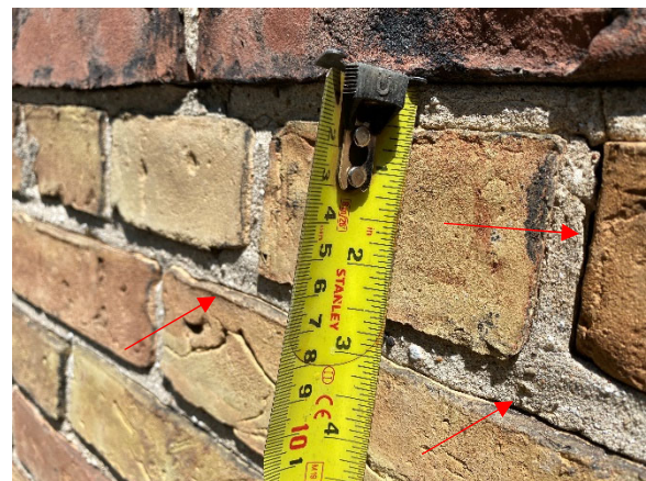
Open Mortar Joints Open joints allow water ingress
