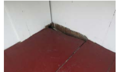
4.2 PAINT LINE VISIBLE ON SOUTHWEST CORNER BELOW PEW ON CHOIR BALCONY
