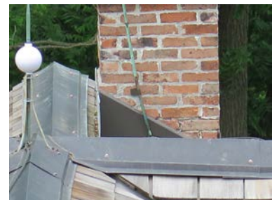
8.4 UNSYMPATHETIC FLASHING AT CHIMNEY
