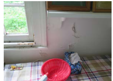
4.5 PEELING PAINT ON SOUTH WALL OF VESTRY
