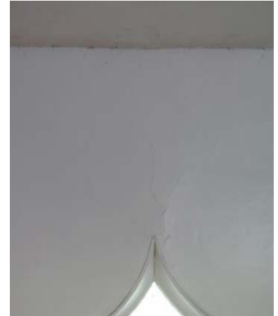
3.1 CRACK ABOVE WINDOW HAS PROGRESSED SINCE THE 2016 REPORT
