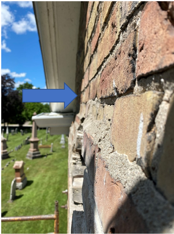
Existing Wall Condition Looking North Wall steps outward from 24" below eave and sweeps inward towards soffit panel. Slope inward ranges from 2" to 3"
