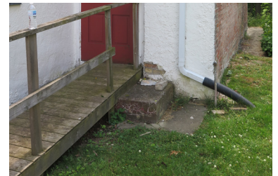
2.3 ACCESSIBILITY RAMP SHOWING ALGAL STAINING
