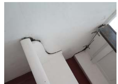
3.4 GAP AND METAL TIES AT NORTH BALCONY AND EAST WALL
