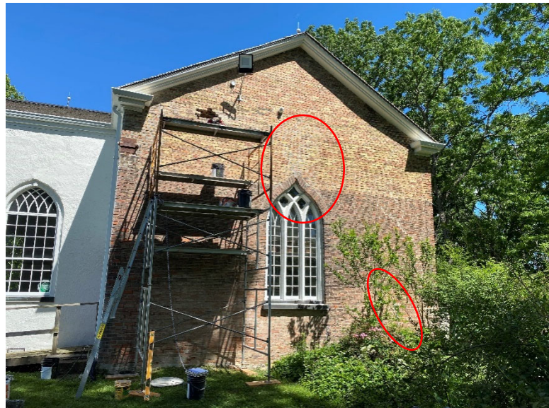
West Elevation Harder denser mortar locations
