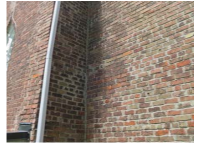
6.4 BRICK BUCKLING AT EXTERIOR CORNER ON SOUTH WALL
