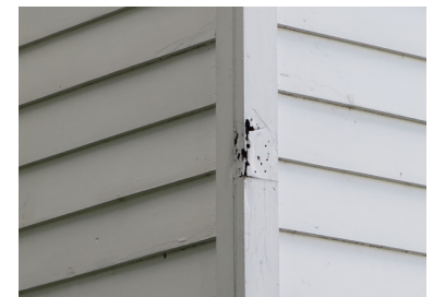
6.1 WOOD SIDING DAMAGED AT BOTTOM CORNERS AND HALF WAY UP TOWER
