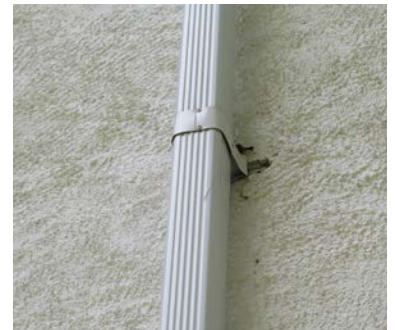
6.5 PREVIOUS DOWNSPOUT CONNECTION EMBEDDED IN STUCCO
