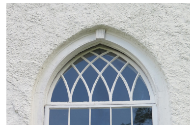
5.1 NAVE WINDOW FRAMES IN NEED OF REPAIR
