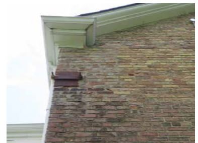
6.9 BUCKLING BRICKWORK AT WEST TRANSEPT GABLE
