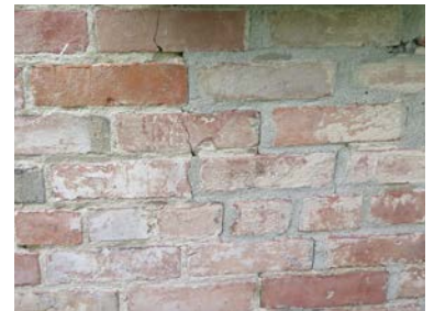
6.6 STEPPED CRACKING AT WEST TRANSEPT WINDOW
