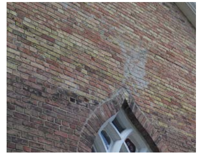
6.8 CEMENT PARGING ABOVE EAST TRANSEPT WINDOW
