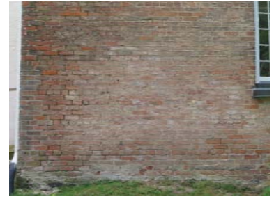
6.7 SPALLED BRICK AT NORTHWEST TRANSEPT CORNER
