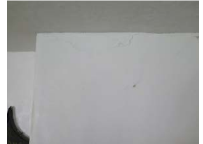
4.1 CRACKS ALONG SOUTH WALL OF CHOIR BALCONY AT THE CEILING
