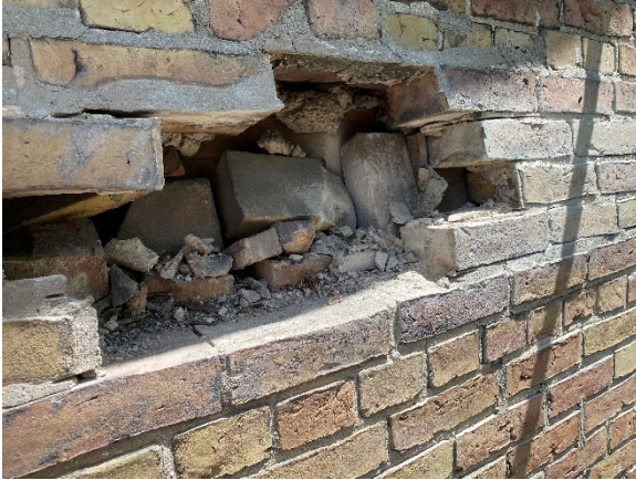
Masonry Opening Random brick loose laid in inner core
