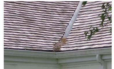
7.2 DEBRIS ACCUMULATING IN ROOF VALLEYS
