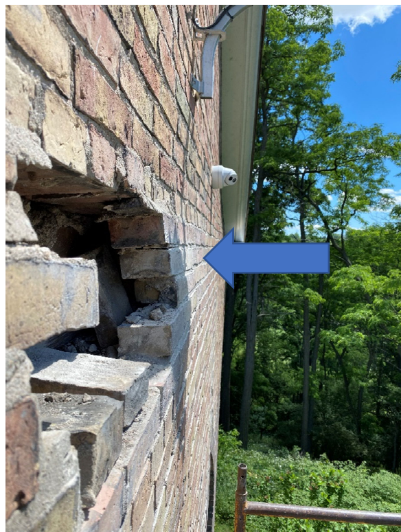
Existing Wall Condition Looking South South line has a more subtle sweep
