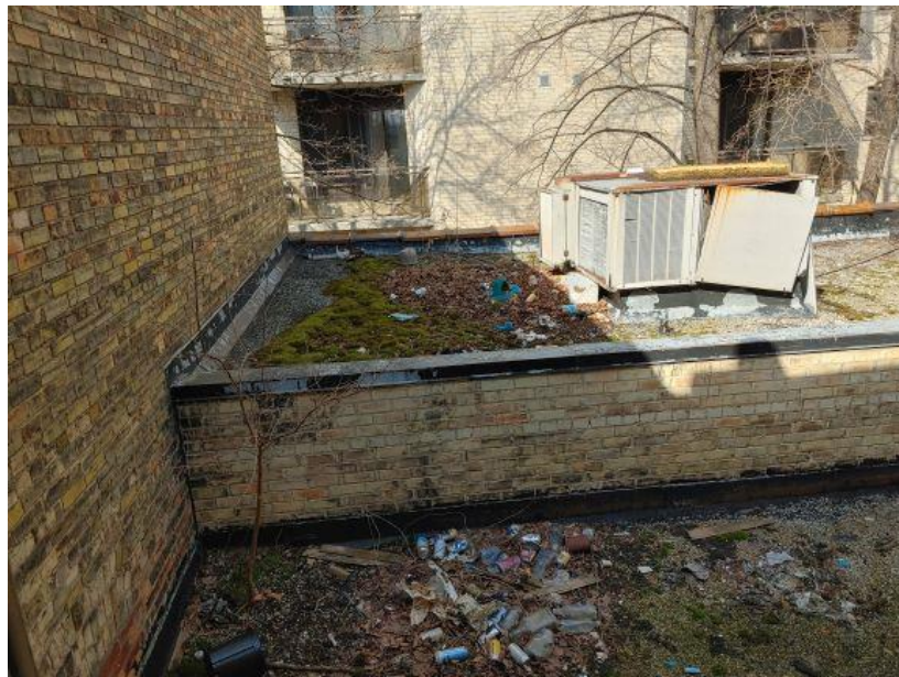
Photograph 2 – Low Roof: Debris and Abandoned Roof top Unit
