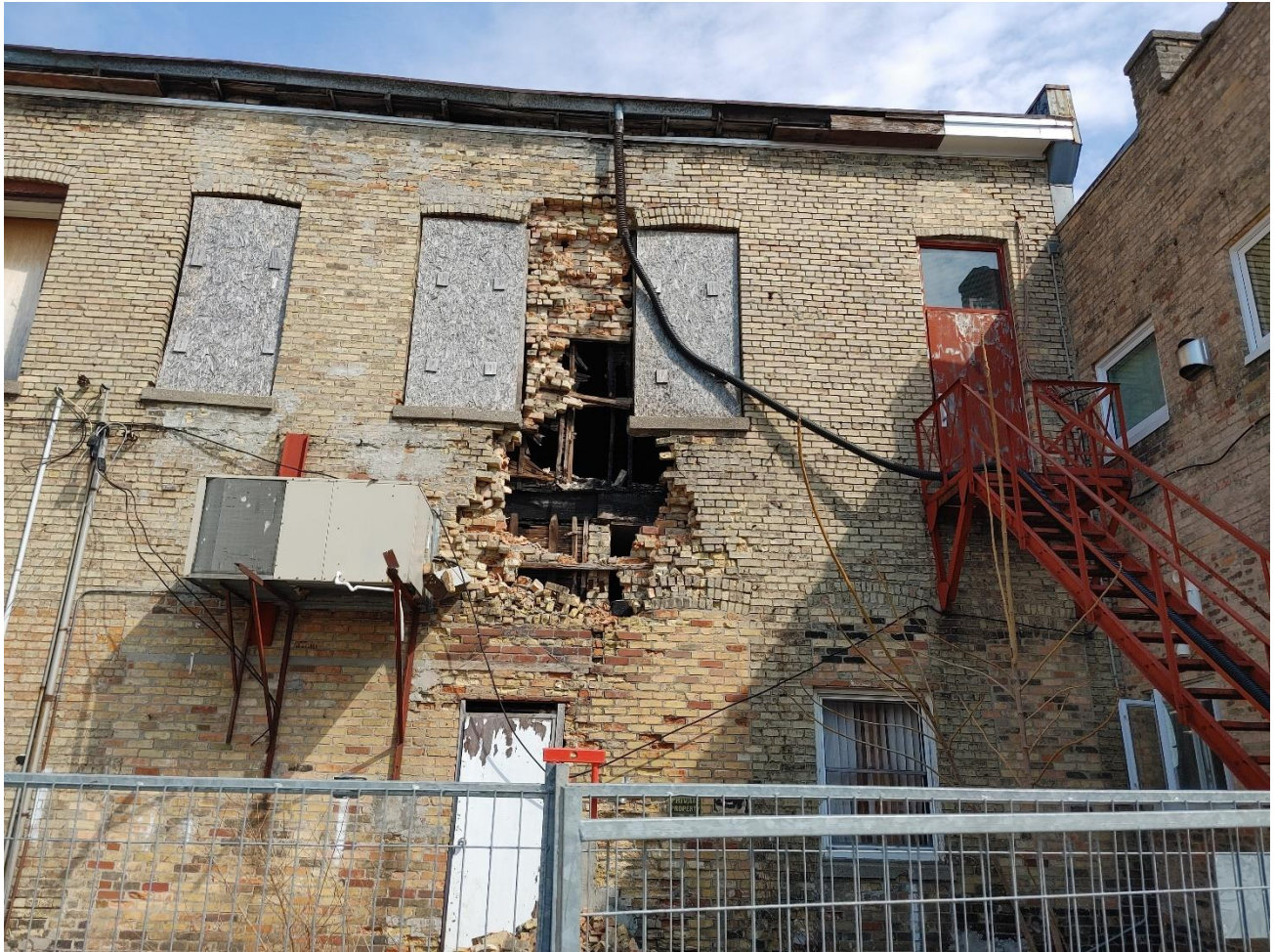
Photograph 1 – Back of Building: Collapse of Brick Facade
