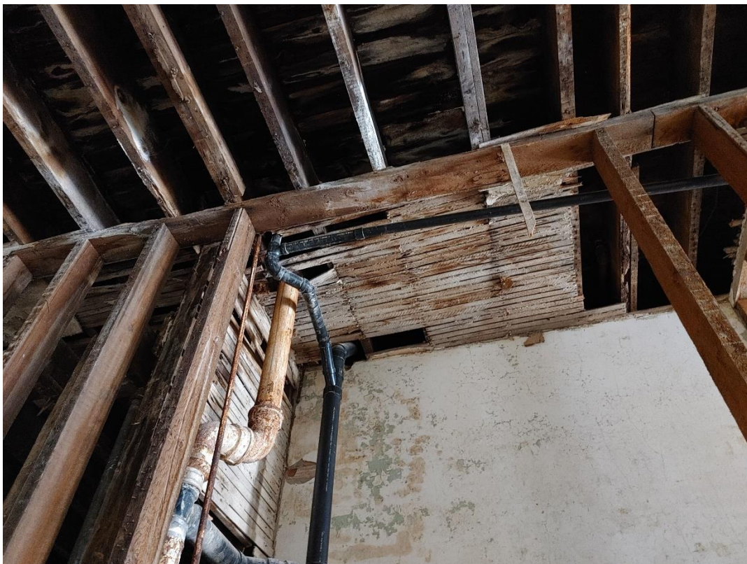
Photograph 14: Opening through Load Bearing Wall (No Lintel, No Blocking)
