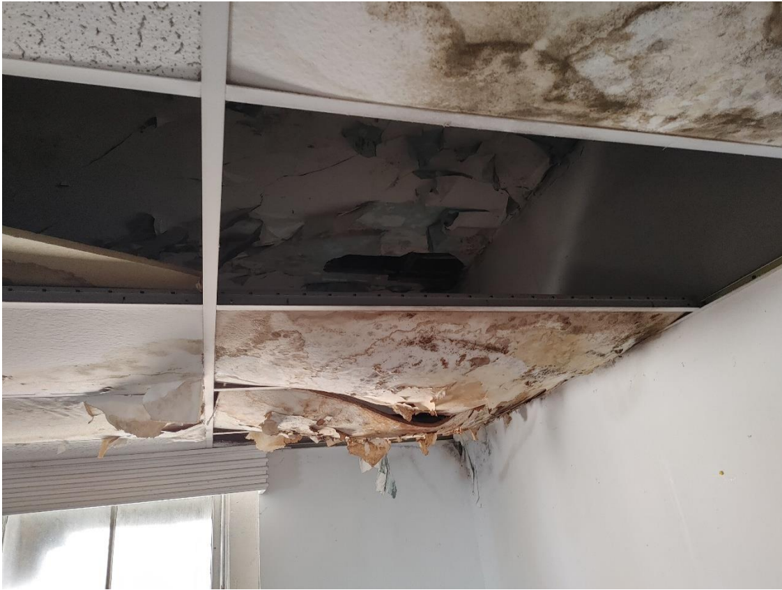
Photograph 11: Evidence of Many Roof Leaks
