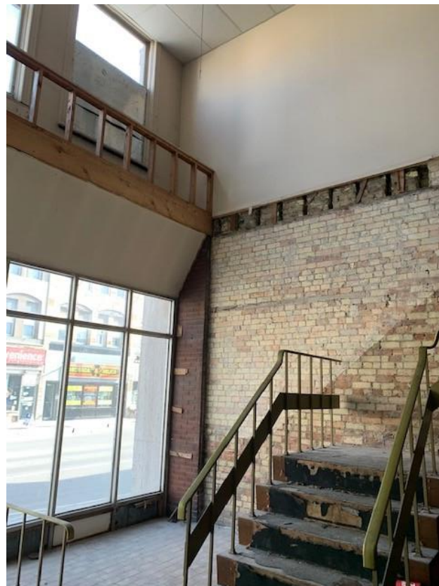
Photograph 6 – Renovation in Unit 360: Level 2 Framing Removed – Masonry Wall Unbraced at Level 2
