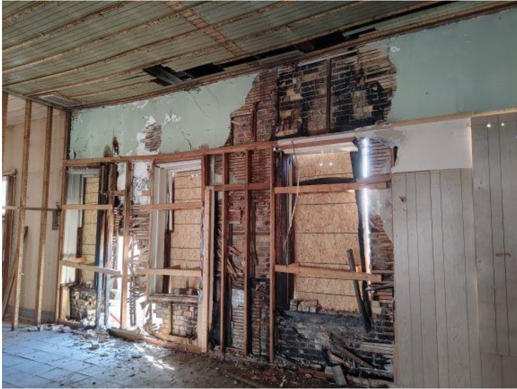
Photograph 7: Additional Façade Collapses on Back of Building
