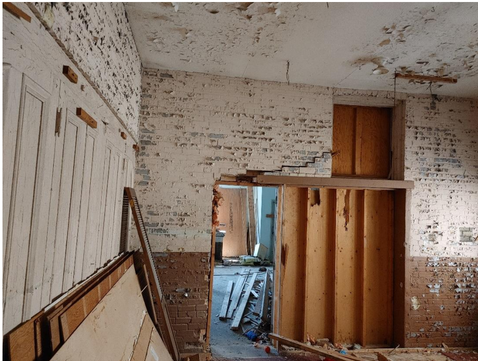
Photograph 12: Opening Through Brick Wall Without Proper Lintel
