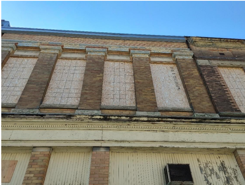
Photograph 9: Boarded Up Windows with Plywood at Frontage of Building
