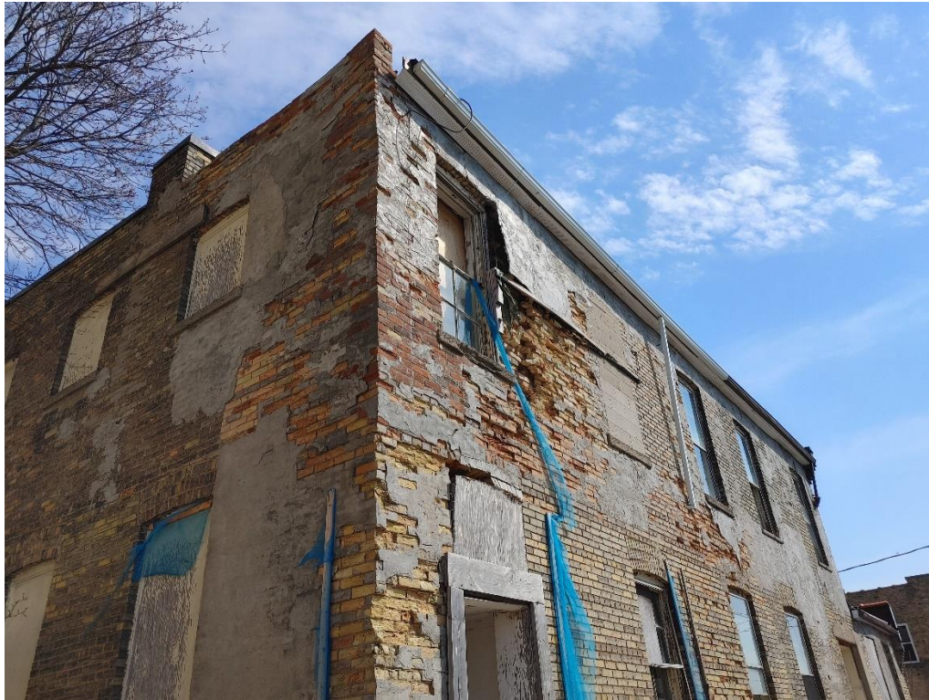
Photograph 13: Large Damage to Back of Building Brick Façade
