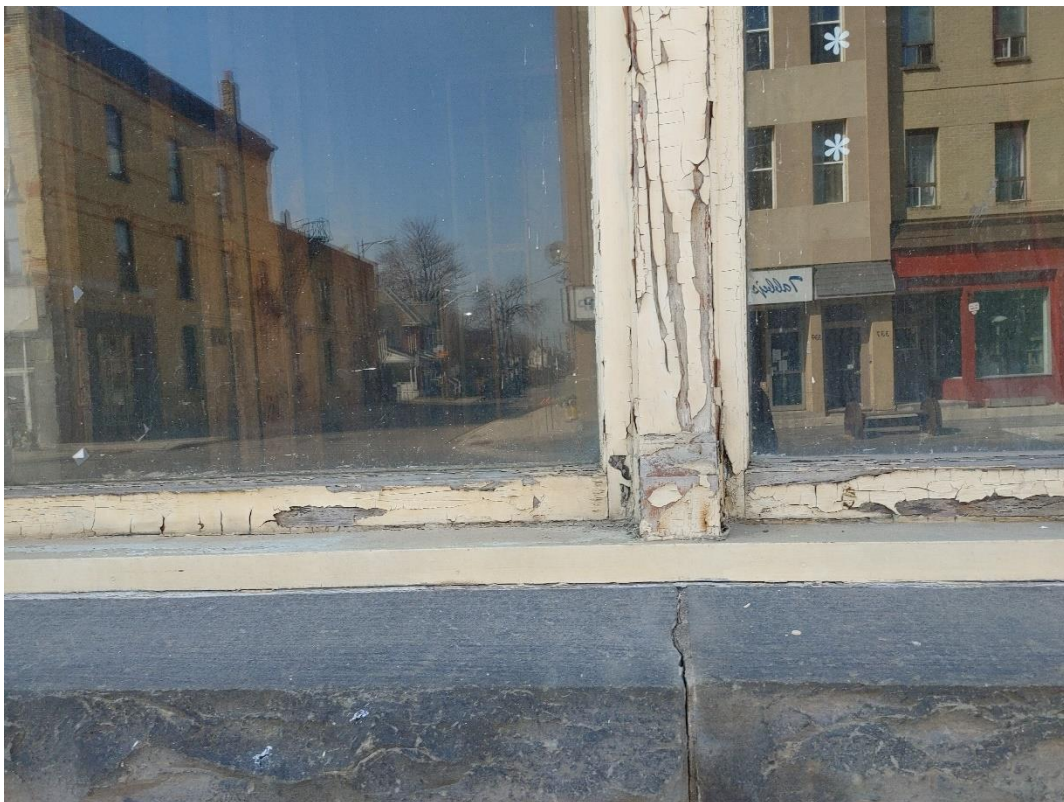
Photograph 10: Damaged window frame (Typical)
