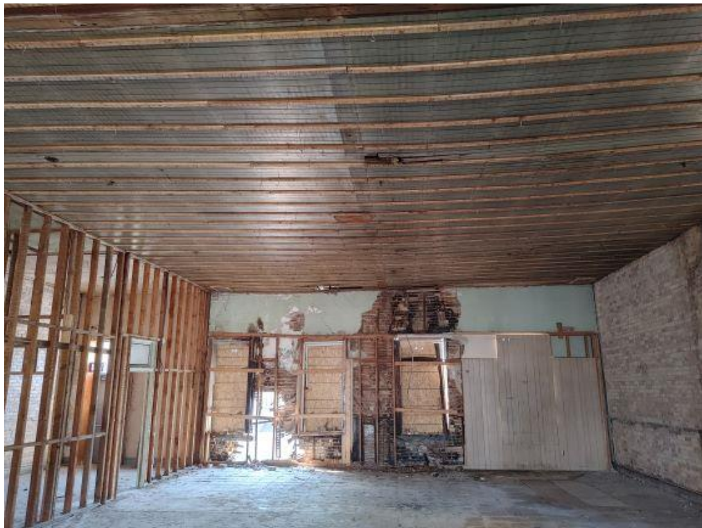
Photograph 8: Roof Framing Sagging at Unit 360 and Roof Leak at Midspan
