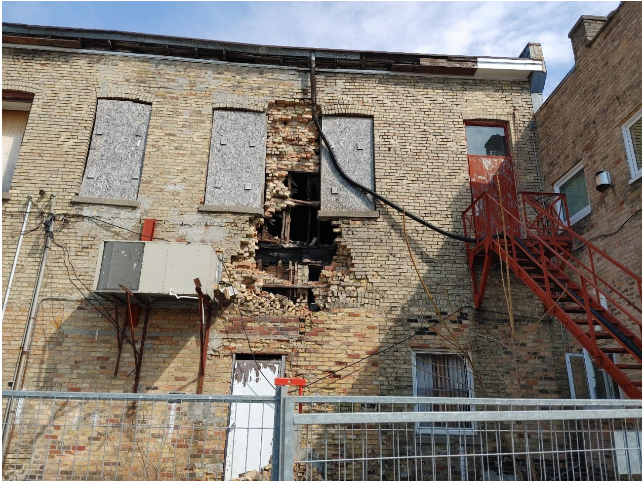
Photograph 1 – Back of Building: Collapse of Brick Facade
