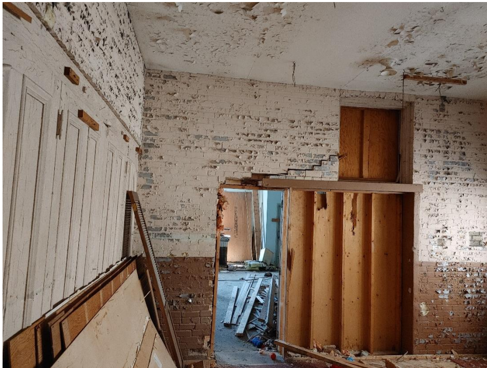
Photograph 12: Opening Through Brick Wall Without Proper Lintel
