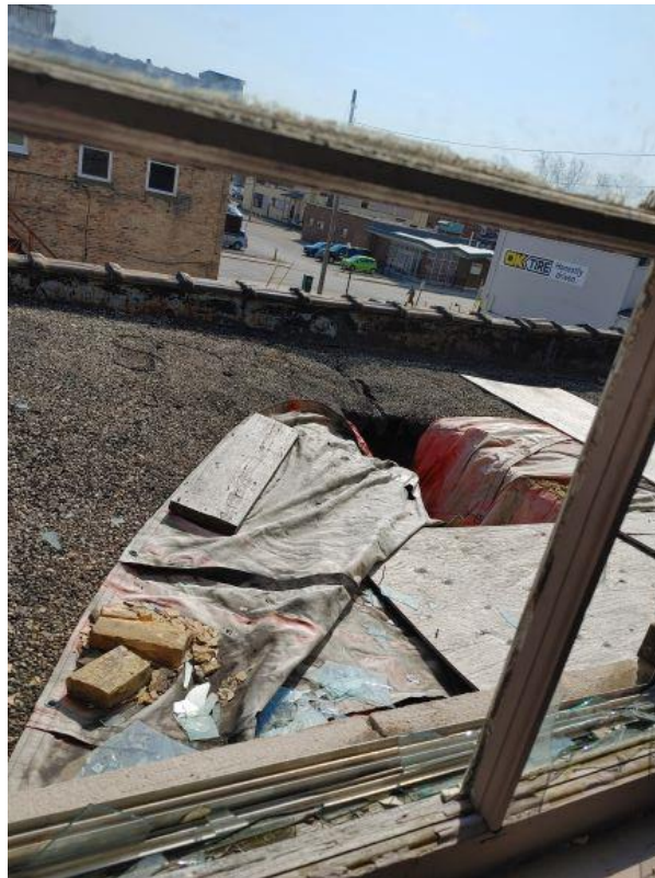
Photograph 3 – Roof Collapse on Low Roof
