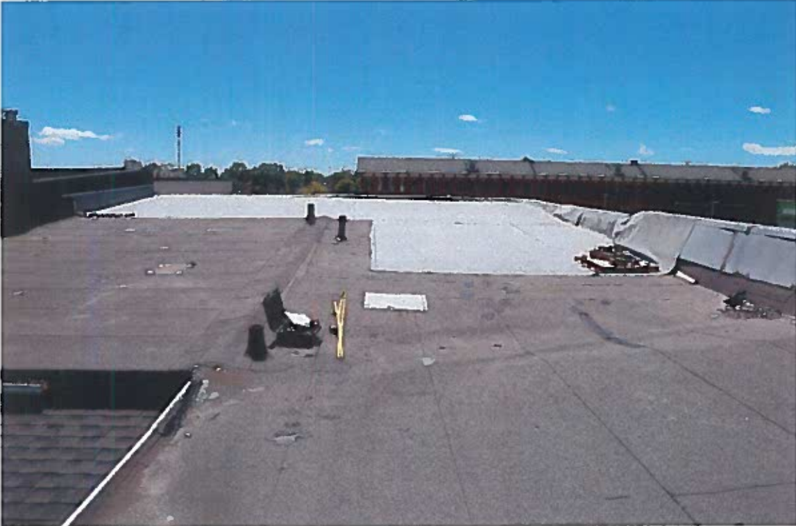
Figure 5. The South section of the roof covered the damaged areas and South and West parapet walls with membrane
