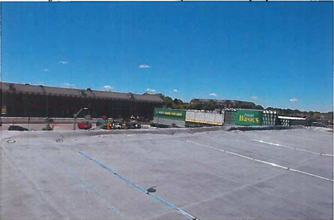
Figure 8. The West section of the roof adjacent to the South parapet wall
