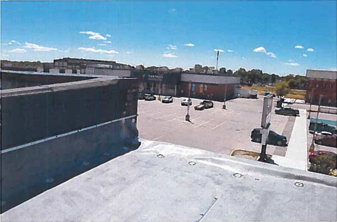
Figure 7. The East section of the roof adjacent to the South parapet wall
