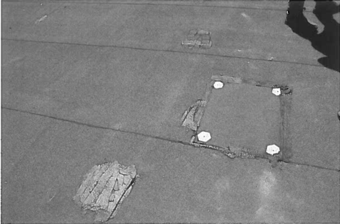
Figure 9. The patched section of the roof at the broken and displaced brick chimney location
