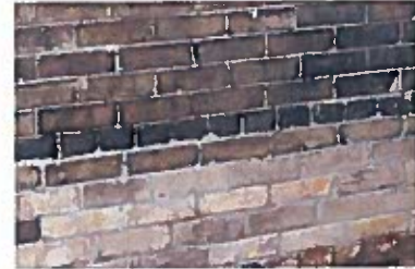
Colour difference due to accumulation of dirt on brick. Cleaning for aesthetics reasons may be considered.
