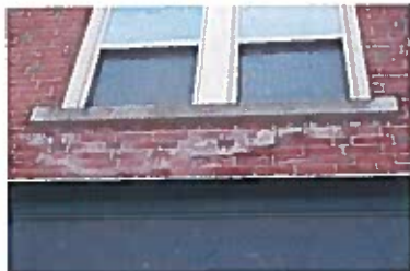
Efflorescence under window due to improper water drainage can cause damage to masonry. Consider methods to reduce water damage.
