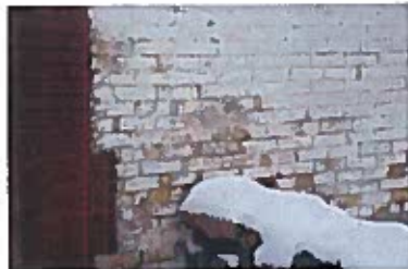
Paint in bad condition on a side of a building, the brick underneath is in very bad condition.
