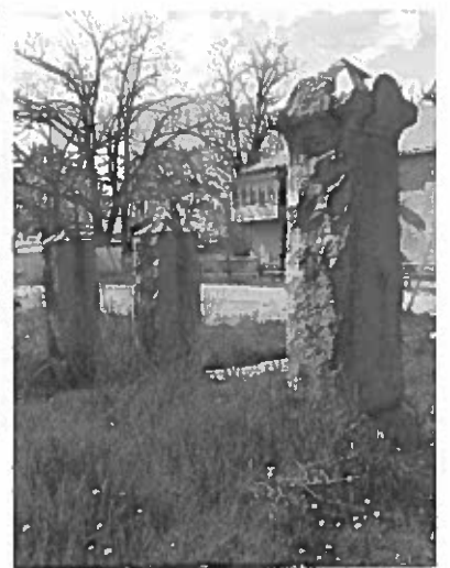
06 Existing condition of the west gate posts at the sidewalk entrance prior to the reinstatement of fencing, gates, lanterns and plaques (EPA, 2018)
